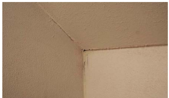
Figure 36: Cracks at the corners.
