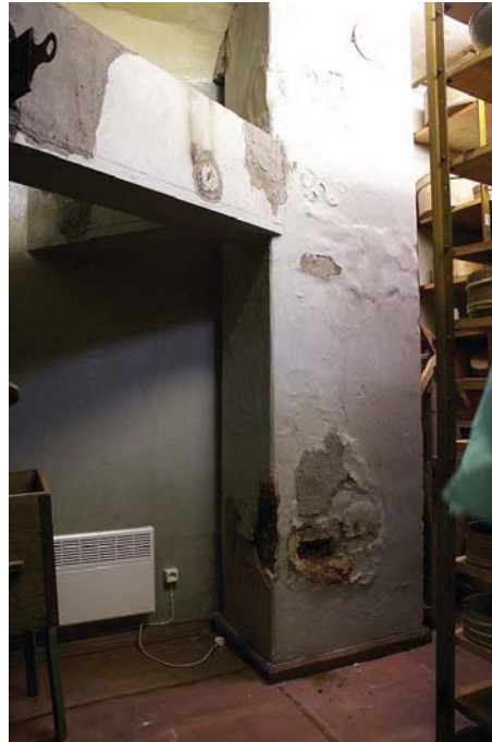
Photo 6: Humidity and mould problem (ground floor).
