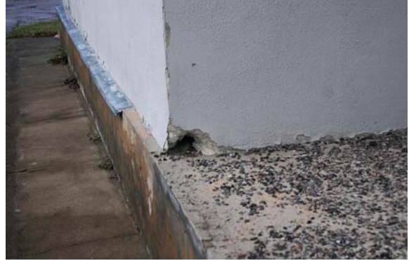
Figure 34: Hole in the wall of the building.
