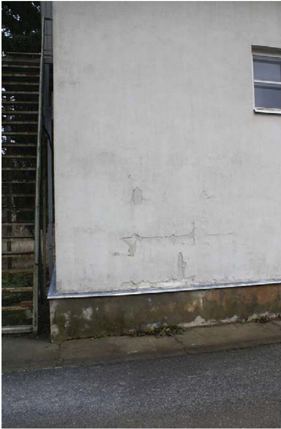
Photo 21: Humidity problem and algae growing on the outside of the building.
