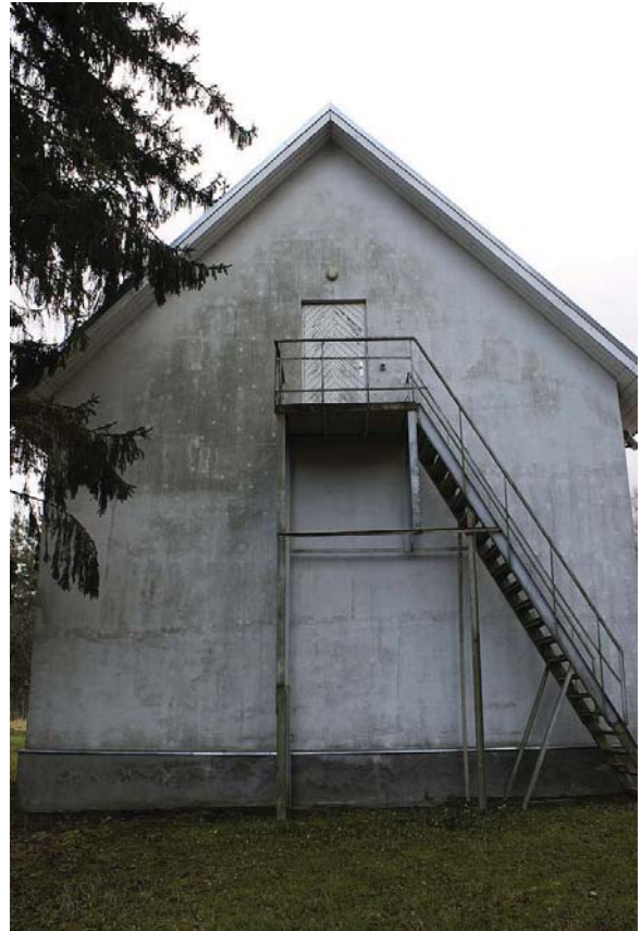
Photo 22: Humidity problem on the back side of the building.
