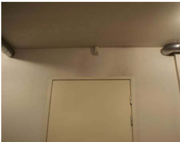
Photo 23: Possible mould problem
