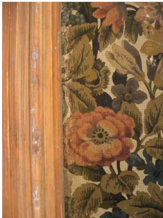
Figure 101. Missing areas in the wallpaper of the Puurmani manor's dining-room were integrated into the rest with the help of modelling lines in matching tones.
