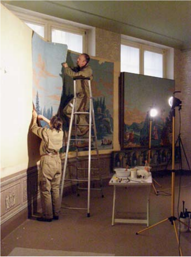
Figure 81. If the bond between the wall and wallpaper is not strong enough it could be removed mechanically by carefully working from behind with a plastic or hord spatula. Photo was taken during the relocation of the wallpaper collection of the German Wallpaper Museum in Kassel.
