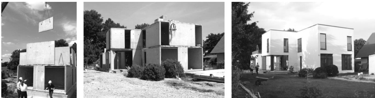
4. Taaskasutatud betoonelementidest elamu. Foto: C. Asam, Recycling prefabricated concrete components – a contribution to sustainable construction, 2007, https://www.irbnet.de/daten/iconda/CIB11828.pdf (vaadatud 13. V 2024).
